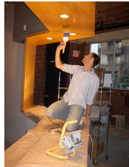
Joseph Pitruzzelli putting the finishing touches on the bar at the DTLA location
